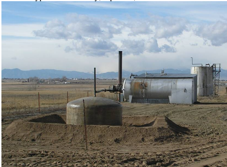
Inset H: Typical tank Battery, separator, and heater
